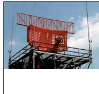
ASR-8 AIRPORT SURVEILLANCE
